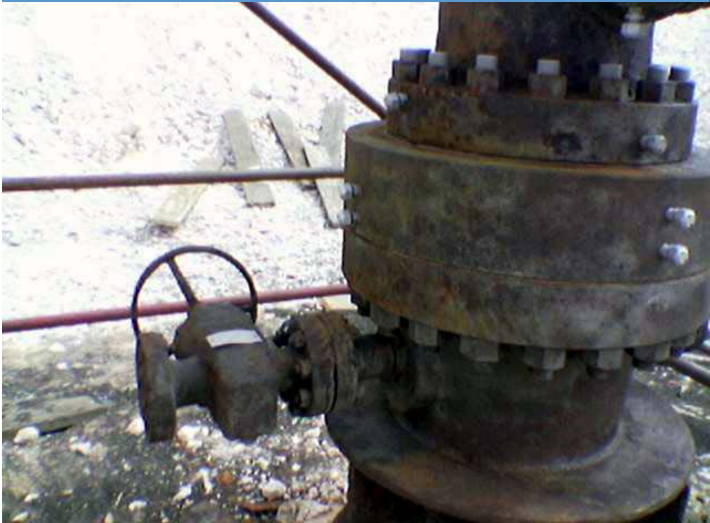
CLOSE-UP OF EXTENSIVE CORROSION
